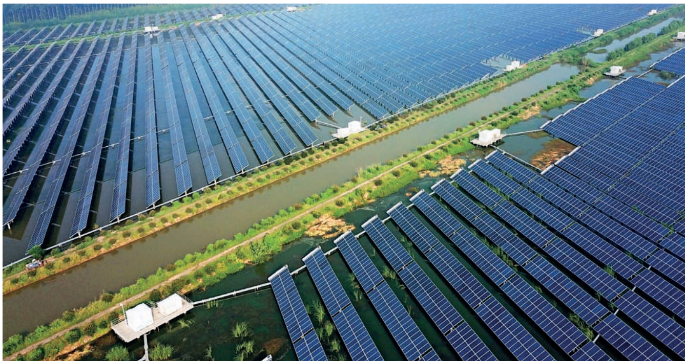
Aerial photo taken on August 9, 2018 shows a photovoltaic power plant built above the fish pond in Yintu Township of Jinhu County, East China's Jiangsu Province. Li Yuze
